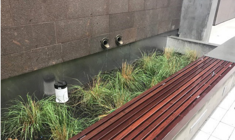
Flow-through planters at the recently completed Mesa Court Towers filter storm water through sand and phytoremediation before reentering the storm drain system.
